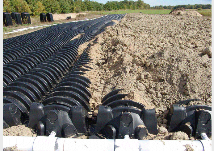
A cluster system being installed in a residential neighborhood (photo courtesy of Infiltrator Systems Inc.).
