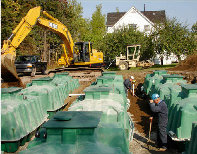
Large subsurface dispersal systems may be regulated as Class V wells under the Safe Drinking Water Act's Underground Injection Control Program. (Source: Premier Tech Aqua)
